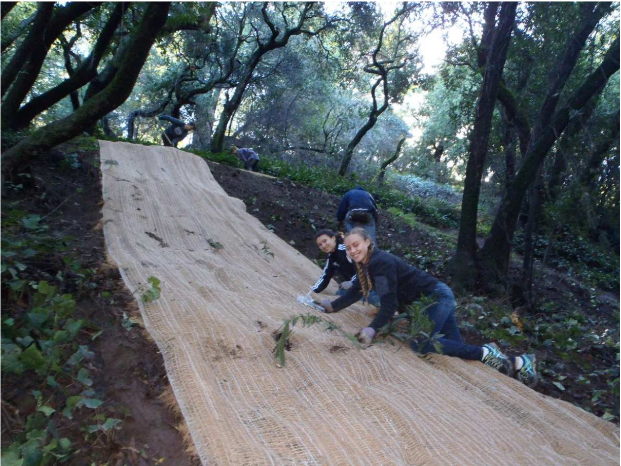
Picture 1: Students from the Piedmont Community Service Crew installing erosion control fabric along the Bridgeview Trail switchbacks in Dimond Canyon
